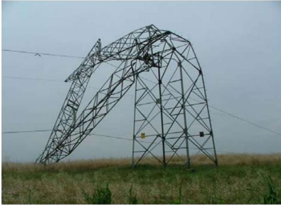
Figure 7.3.: Ruined pillar for high-voltage transmission lines
